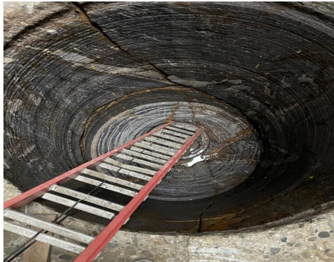
This 9-foot diameter shaft under the George Washington Bridge cored using ECT Core Barrel.
